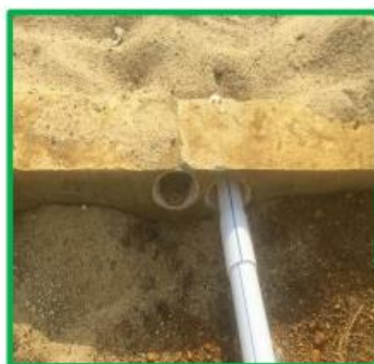
View of conduit
